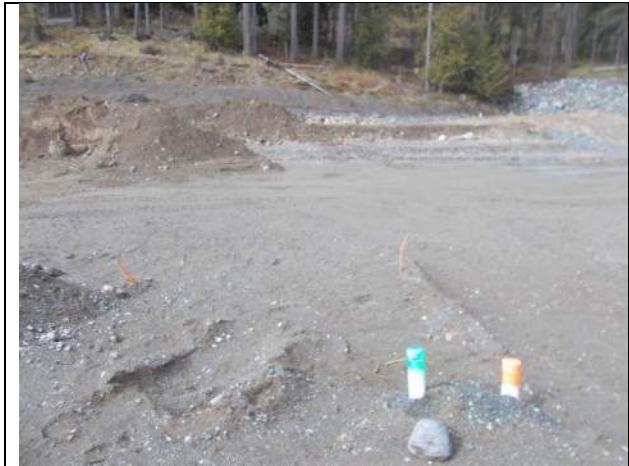
Apr. 1, 2023: Current condition of Lot 49, with pit run sand and gravel exposed as subgrade.
