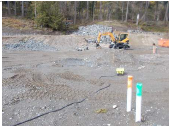
Apr. 1, 2023: Current condition of Lot 52, with pit run sand and gravel exposed as subgrade.
