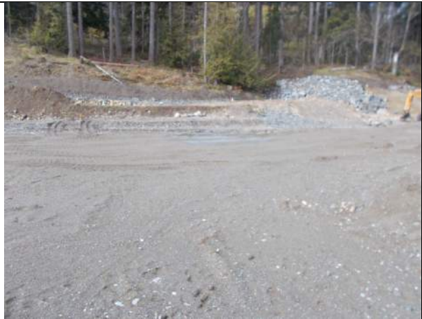
Apr. 1, 2023: Current condition of Lot 50, with pit run sand and gravel exposed as subgrade.
