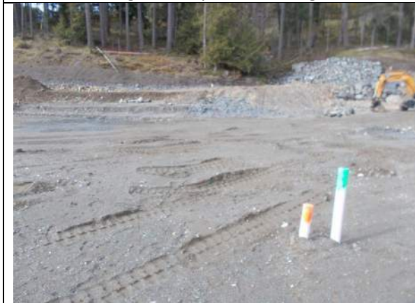
Apr. 1, 2023: Current condition of Lot 51, with pit run sand and gravel exposed as subgrade.
