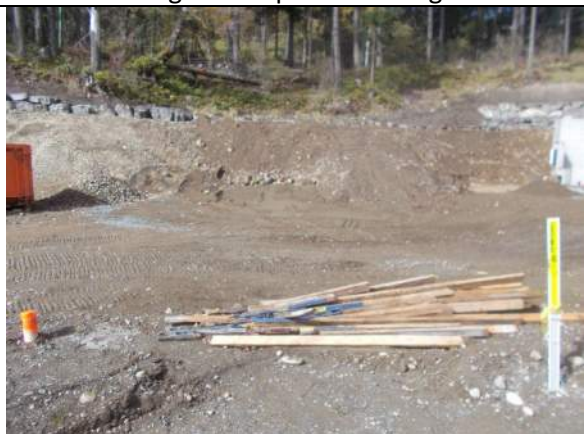
Apr. 1, 2023: Current condition of Lot 54, with pit run sand and gravel exposed as subgrade.
