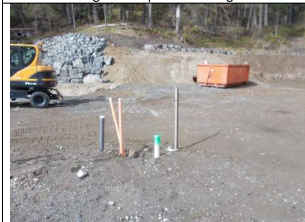
Apr. 1, 2023: Current condition of Lot 53, with pit run sand and gravel exposed as subgrade.
