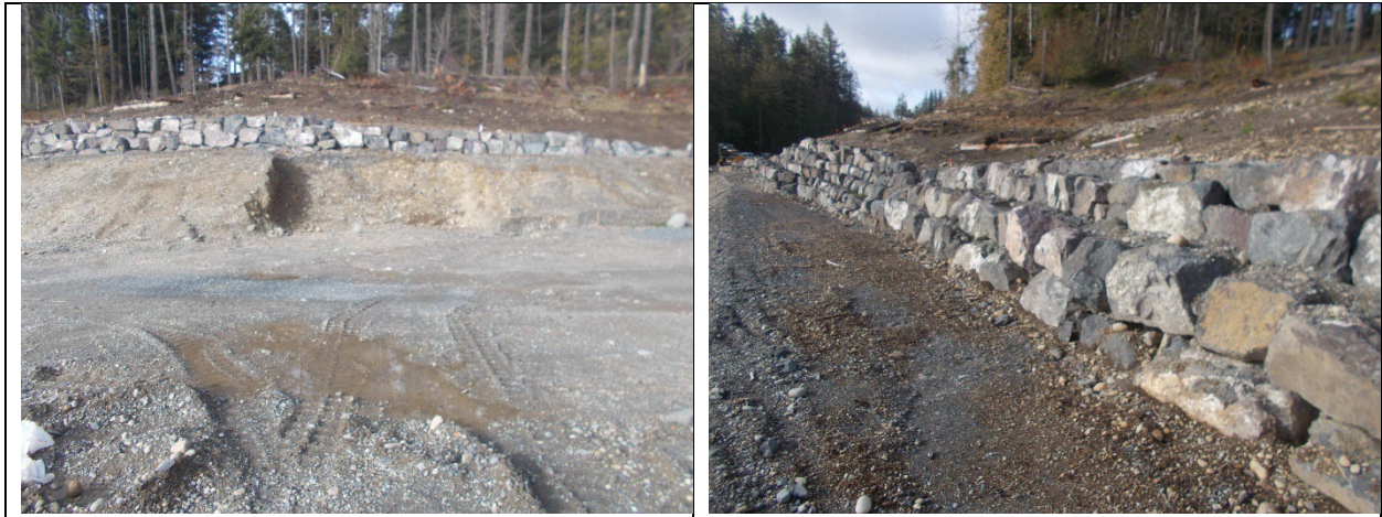
Mar. 15, 2023: Current condition of Lot 43, with house site excavated into pit run sand & gravel.
