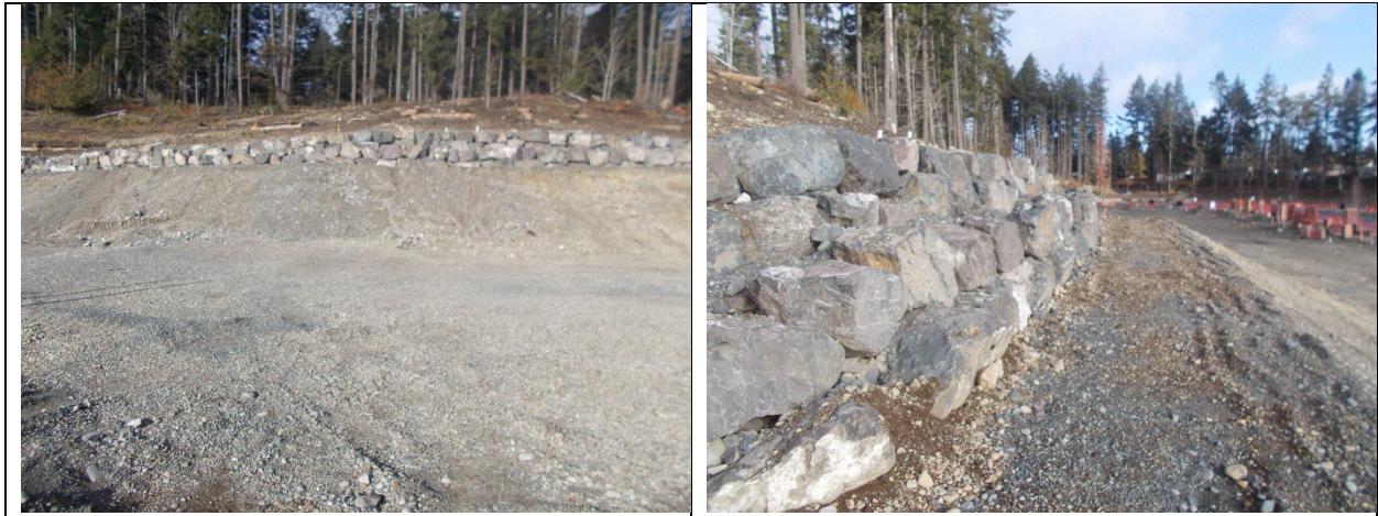
Mar. 15, 2023: Current condition of Lot 41, with house site excavated into pit run sand & gravel.
