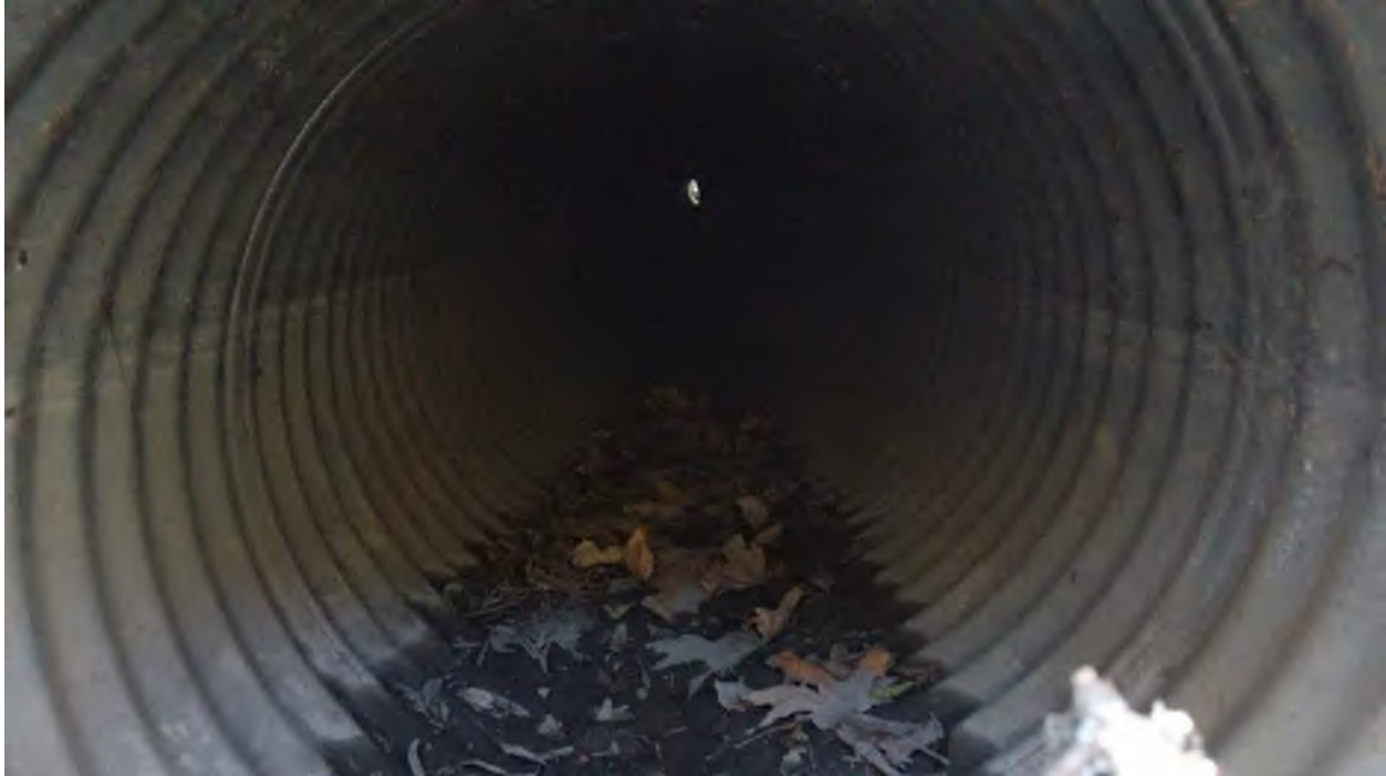
Figure 10. View into the culvert (Figure 8) showing the narrow ribbon of sediment that lines the bottom of the culvert under VMP. Note the absence of a rust line on the bottom sides of the CSP culvert, indicating that there are only periodic low volumes of runoff flowing in the culvert. The sediment lining the bottom of the culvert has settled out to a depth equivalent to the height of the berm (Figure 9) obstructing flows through the culvert. The berm obstructing flow through the culvert results in runoff in the culvert becoming stagnant with sediment transport interrupted and sediment settling out. This condition reflects the minimal flows in the drainage catchment upstream of the outlet, indicating there is no stream or natural supply of water sufficient to maintain a sediment free culvert and prevent a berm from forming at the outlet of the culvert (Figure 9). This headwater drainage would be classified as a “stream” under the RAPR but allocated a SPEA under the “ditch” category.
