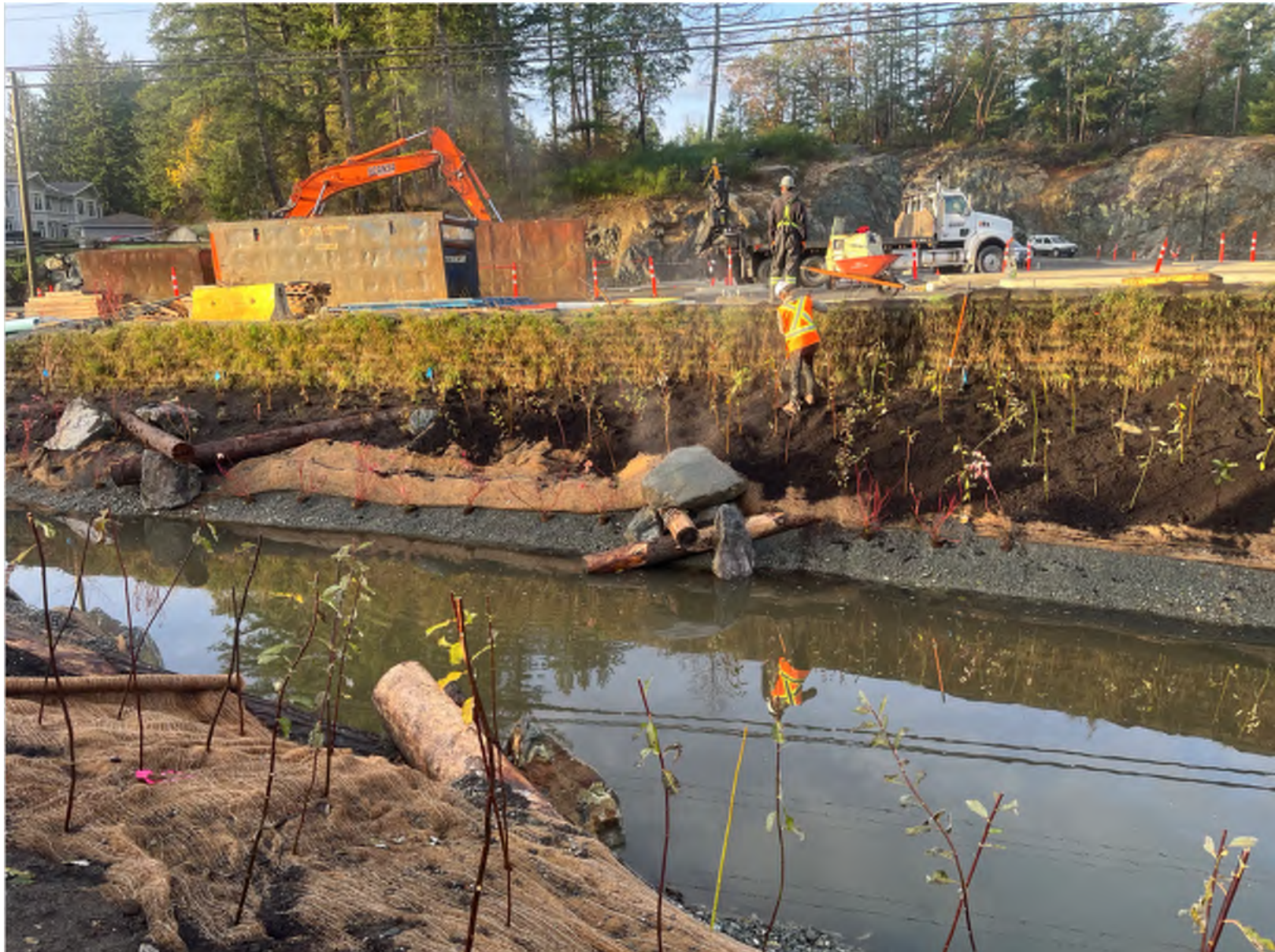
Figure 15. In this image the Flex MSE Vegetated Wall System height is ~1.2m high (yellow arrow). The planting terrace at the base of the wall is ~1.5m high. Note the distinct separation between the vertical wall, the planting terrace, and the gravel terrace.
