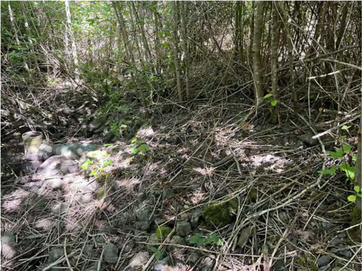
Photo 3. T inlet structure of the upper most treatment pond (yellow arrow). The bottom of the T is almost the same elevation as the invert of the buried culvert. Note the large rock berm separating this treatment pond from the adjacent treatment pond downstream. Blue arrow is the direction of flow. Note the dense blackberry understory with a young red alder tree overstory. Image taken 2022-06-24.
