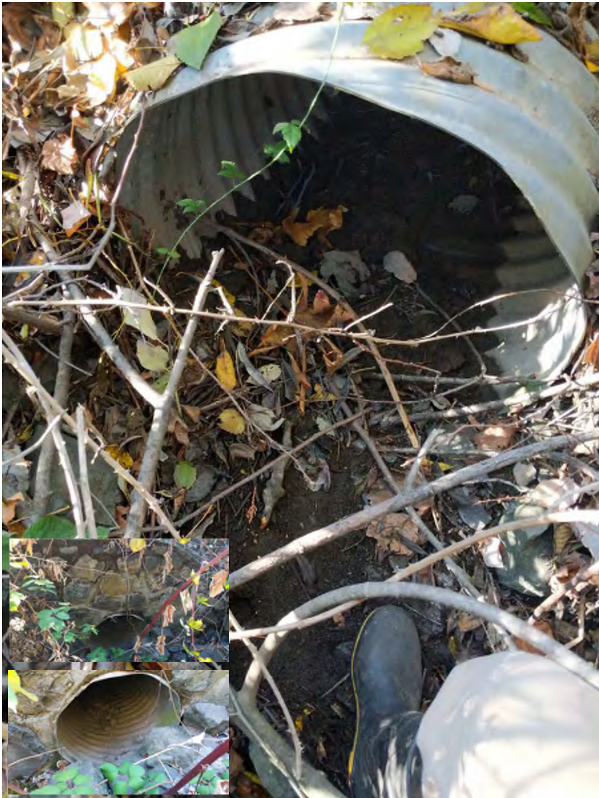
Figure 9. Outlet of the drainage culvert under VMP (Figure 8) showing the blocked outlet consisting of a soil berm which prevents the free flow of periodic, low runoff volumes routed from the west side of VMP into a treatment pond on the east side of VMP. Image inserts of inlet of the culvert, noting that there is no rusted water line or evidence of regular stormwater flow.
