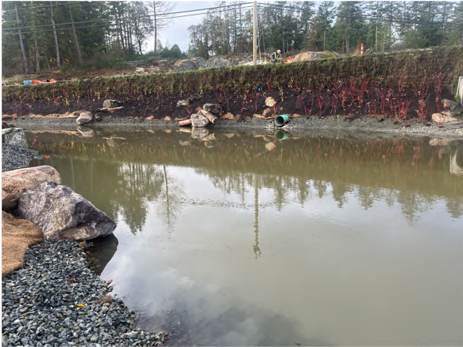
Figure 14. Looking at the vertical Flex MSE Vegetated Wall System (height = ~2m (yellow arrow)). The planting terrace at the base of the wall consists of a sand/gravel lower terrace and a soil terrace above the sand/gravel terrace. The soil terrace is intended as a tree/shrub planting zone.
