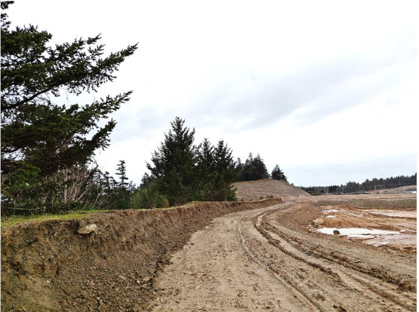
Figure 4 – Edge of service road adjacent eastern bluff
