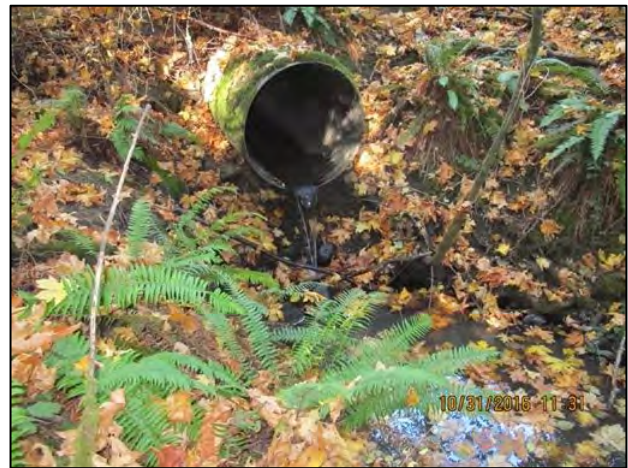
Photo 4 Perched Spruston Creek culvert outlet at Metchosin Road (C. Barlow; October 31, 2016).
