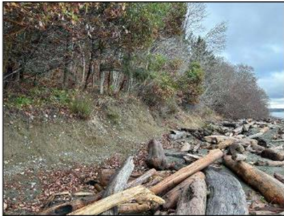
Figure 8 - View of bluff base at location P1
