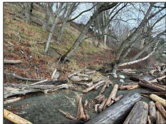
Figure 9 - View of bluff base at location P2
